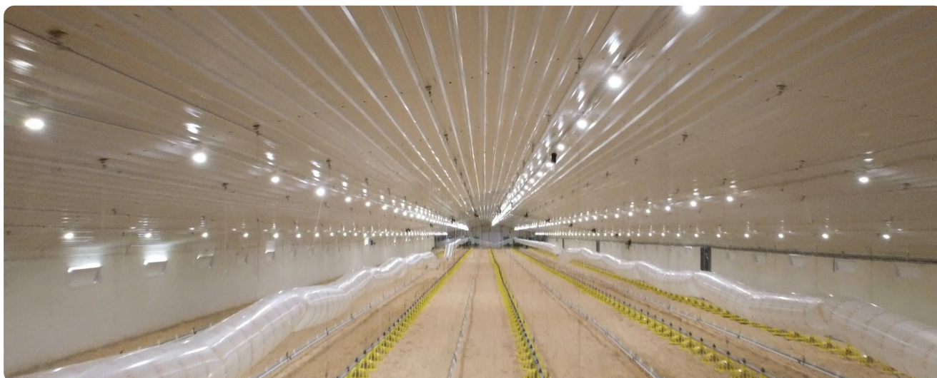
LED fittings along the house (VISIONWARE drone footage). Measure at bird level, never close to the fitting.
